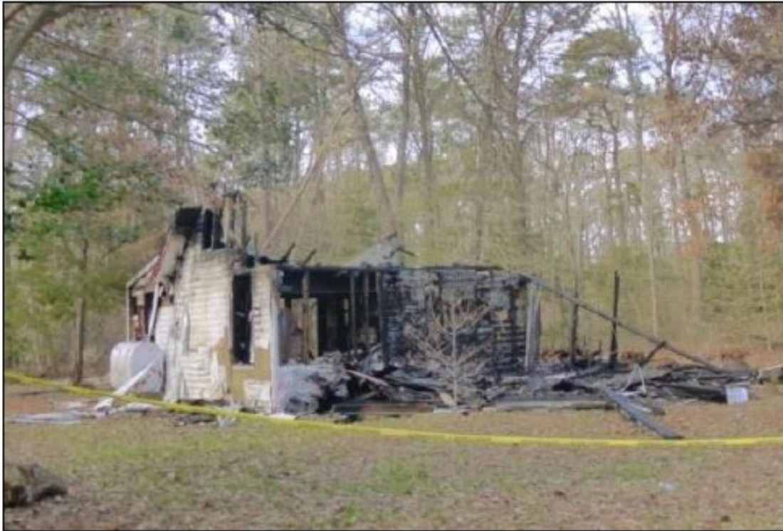
Image #3: The above example image represents damage as the result of a fire.
